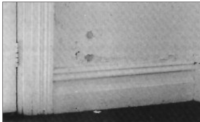
Figure 1. Rising damp lifting finishes.
