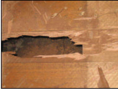
Figure 3. Kalotermes (drywood termite) damage to flooring
