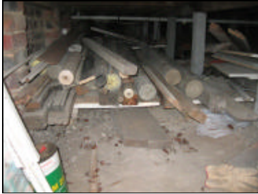
Figure 6. Timber stored in sub floor provides a food haven for foraging termites
