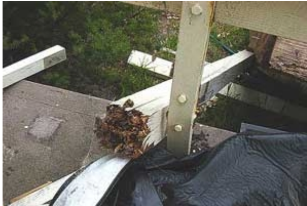
Rotting timber from a balcony collapse
