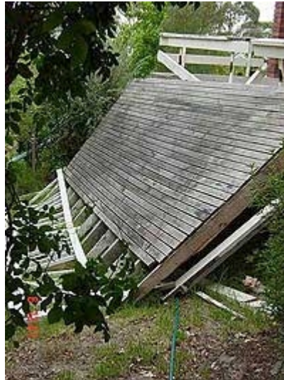
A recent balcony collapse where people were severely injured
