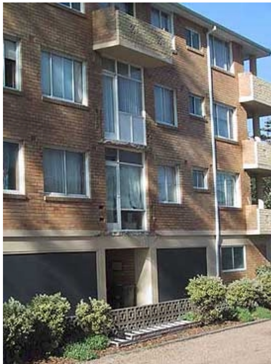
The third floor balcony sheared off the Manly apartment building crashing through the balcony below to the public area at ground level Image courtesy of ACRA
