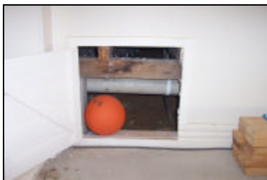
Figure 8. Access hatch cut in an inappropriate place, preventing sub floor access
