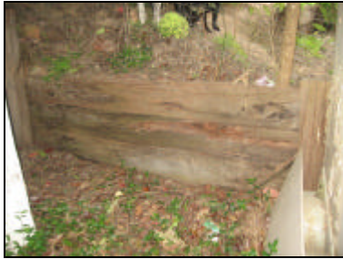
Figure 4. Landscaping timbers in contact with ground
