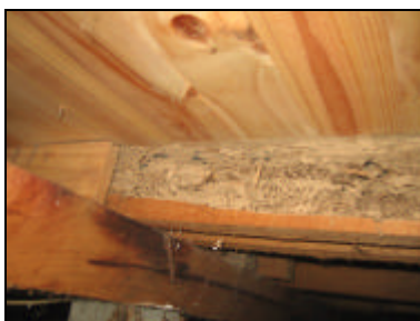
Figure 2. Sub floor bearer damage ( Coptotermes sp )
