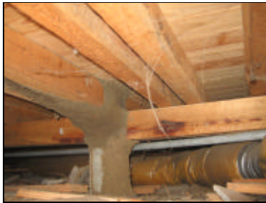
Figure 1. Termite ( Coptotermes sp ) mudding over concrete stumps and bearers
