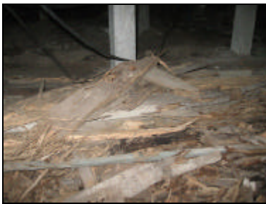
Figure 7. This timber debris left in sub floor has already been attacked by termites
