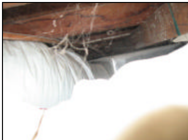
Figure 9. Ducting is a common access problem
