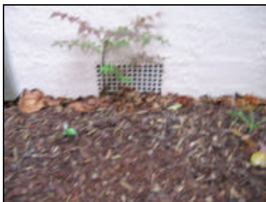
Figure 5. Mulch covering vents
